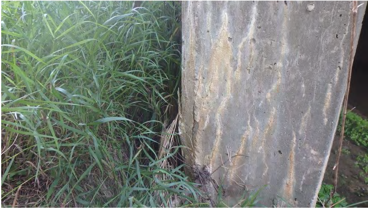
Figure 9 Delamination with chlorides at Southeast Quadrant
