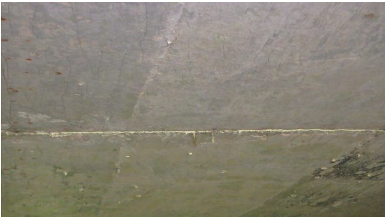
Figure 10 Leakage with chlorides at Joint in North Barrel
