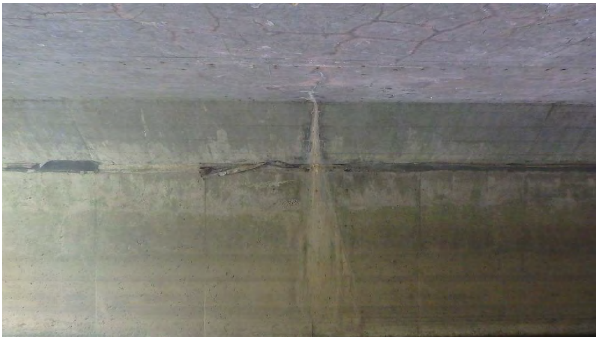
Figure 12 Vertical Crack with Leakage and Chlorides in South Barrel
