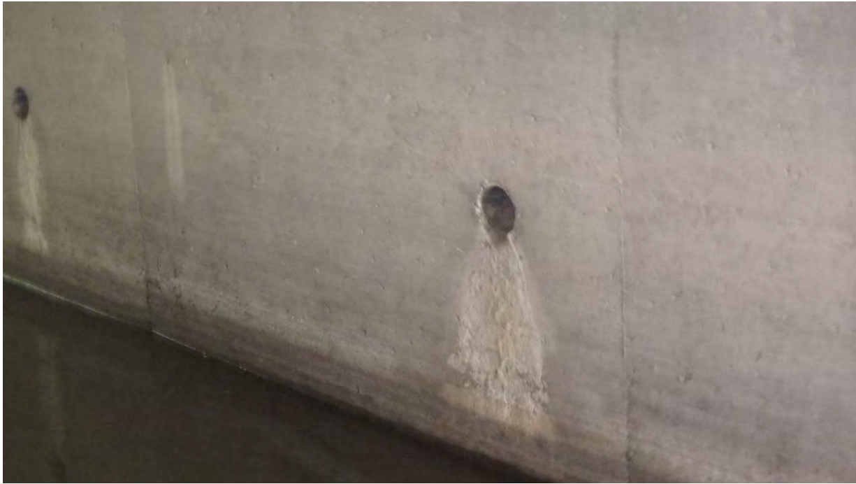
Figure 11 Staining and Deterioration Below Joints in North Barrel
