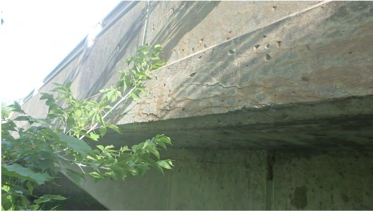
Figure 9 Cracking and Deterioration at Southeast Fascia
