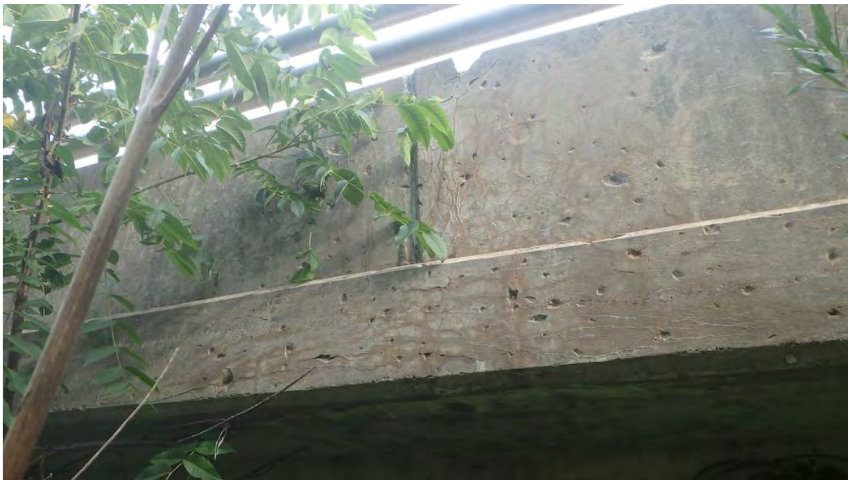
Figure 10 Cracking and Deterioration at Southwest Fascia
