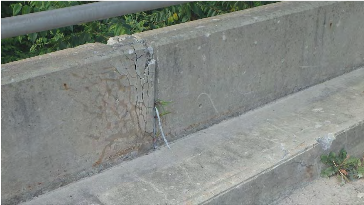
Figure 14 Spalling at Barrier Joints
