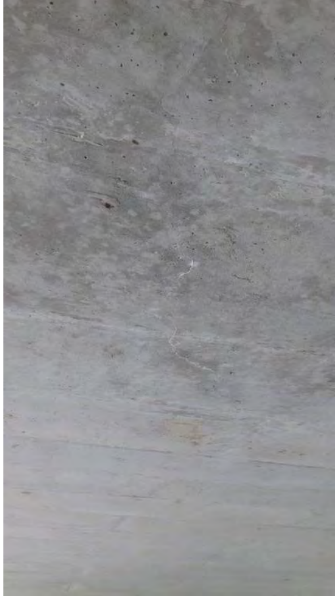
Figure 11 Crack on Soffit with Chloride
