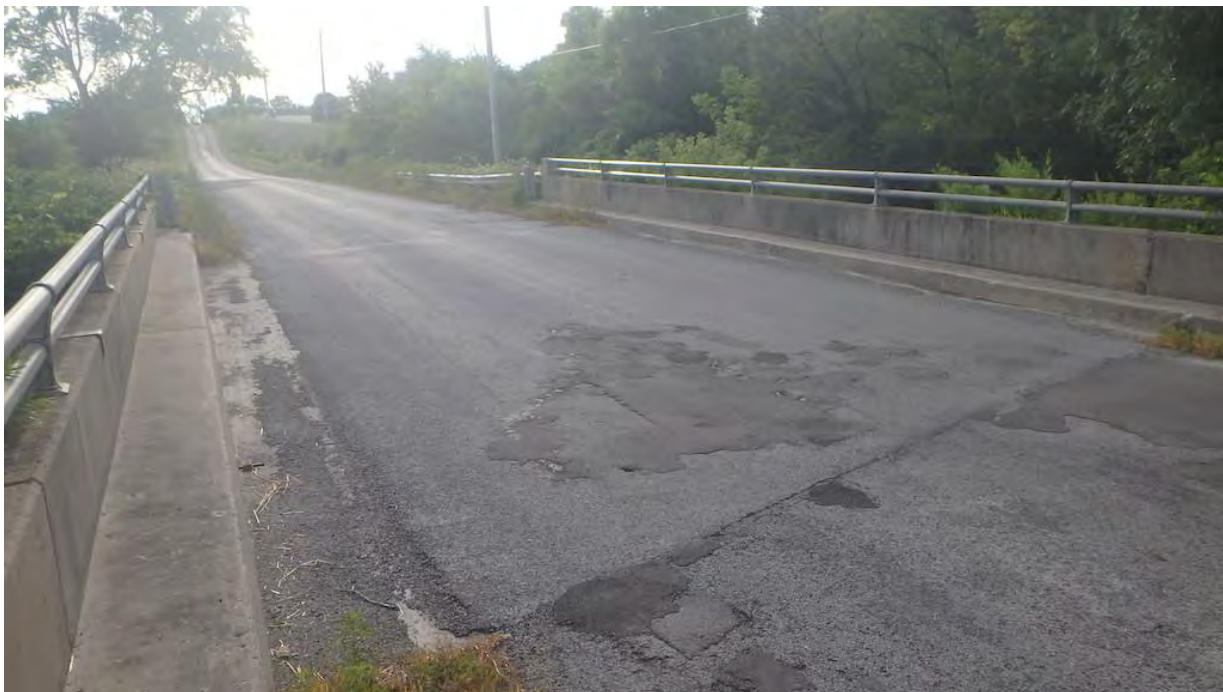
Figure 13 Patched Potholes in Wearing Surface
