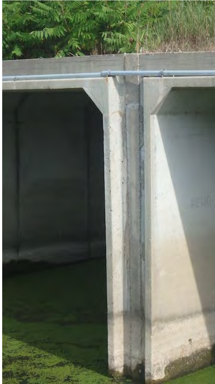
Figure 11 Minor Cracking of Parging Between Outlet Barrels
