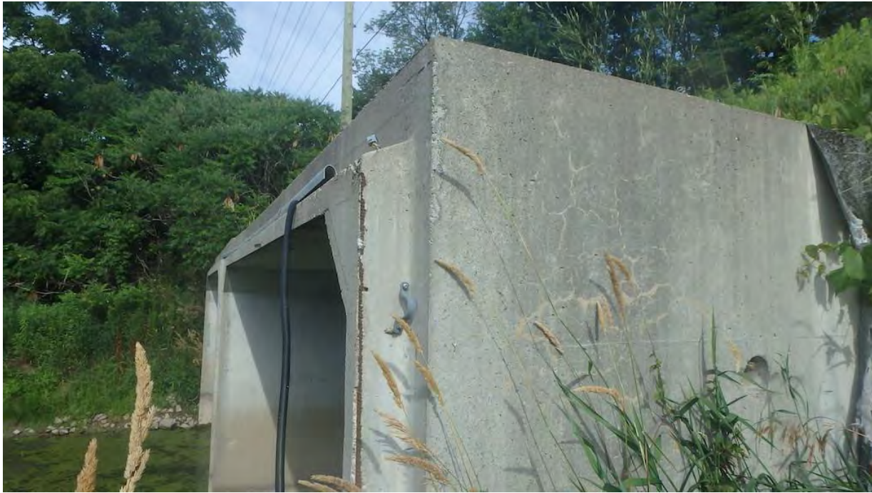
Figure 9 Exposed Rebar and Staining at Southeast Quadrant
