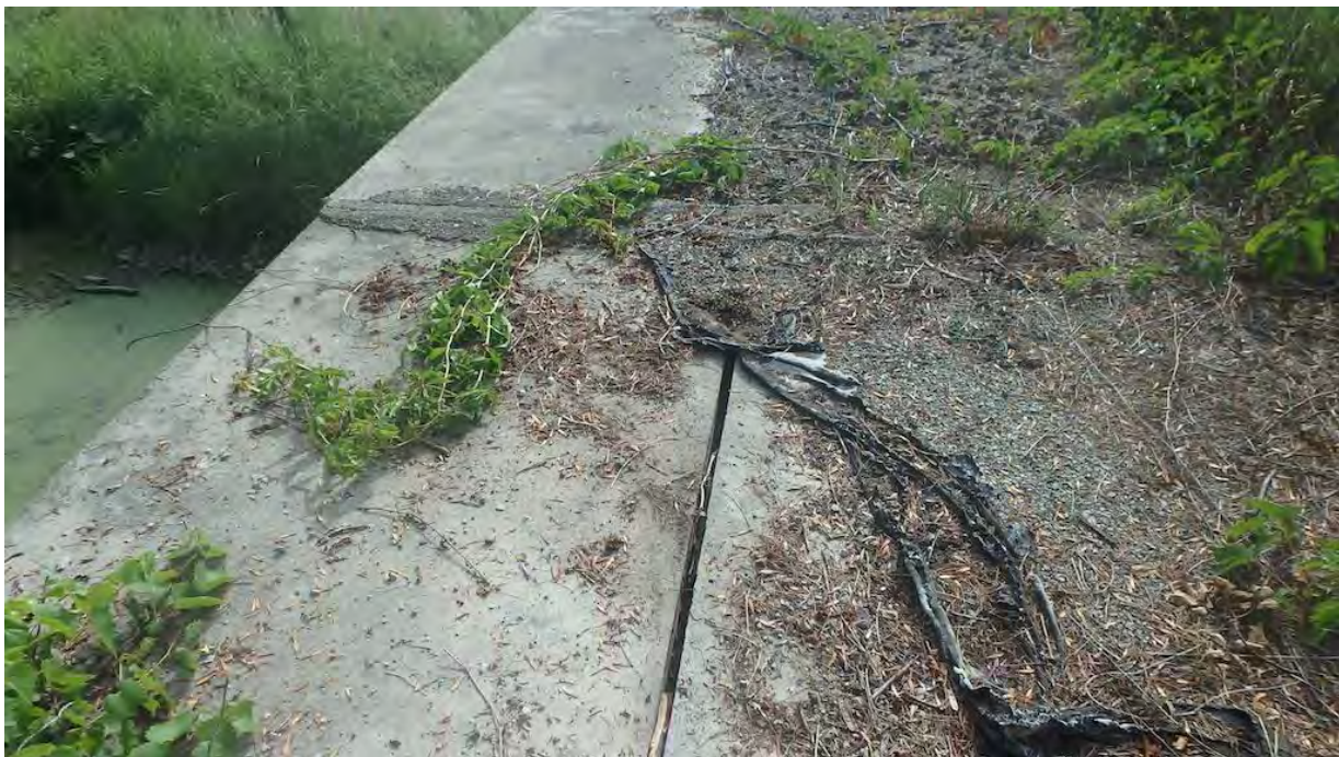
Figure 10 Deterioration of Parking of Joints at Inlet
