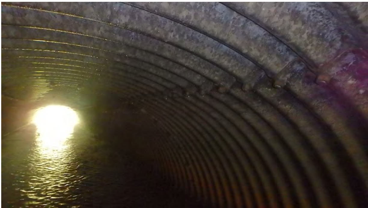
Figure 8 Leaking Multiplate Joints
