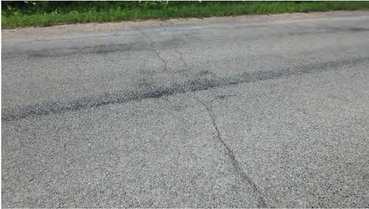
Figure 9 Transverse Crack in Wearing Surface
