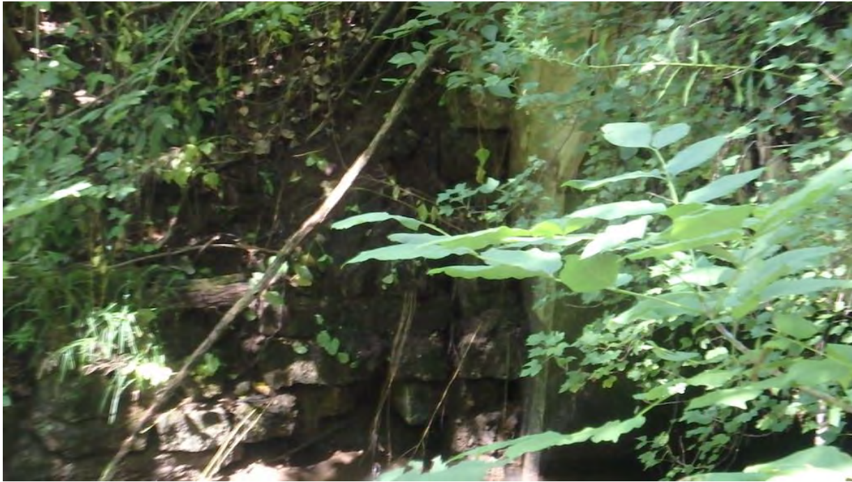
Figure 8 Stone Retaining Wall Deteriorated
