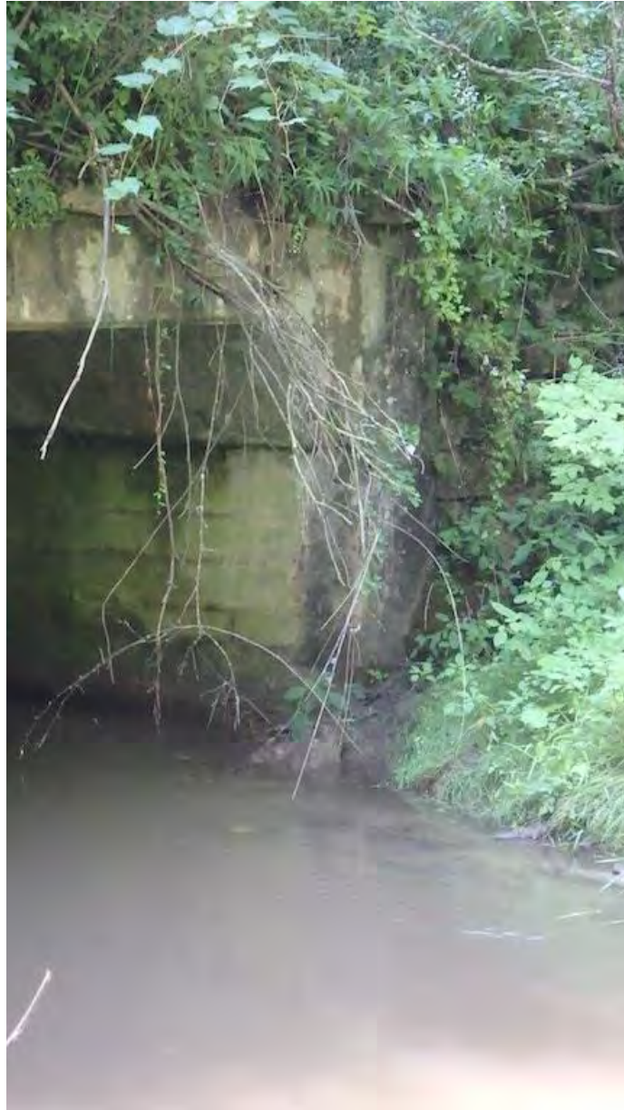
Figure 7 Deterioration at Haunch Construction Joint
