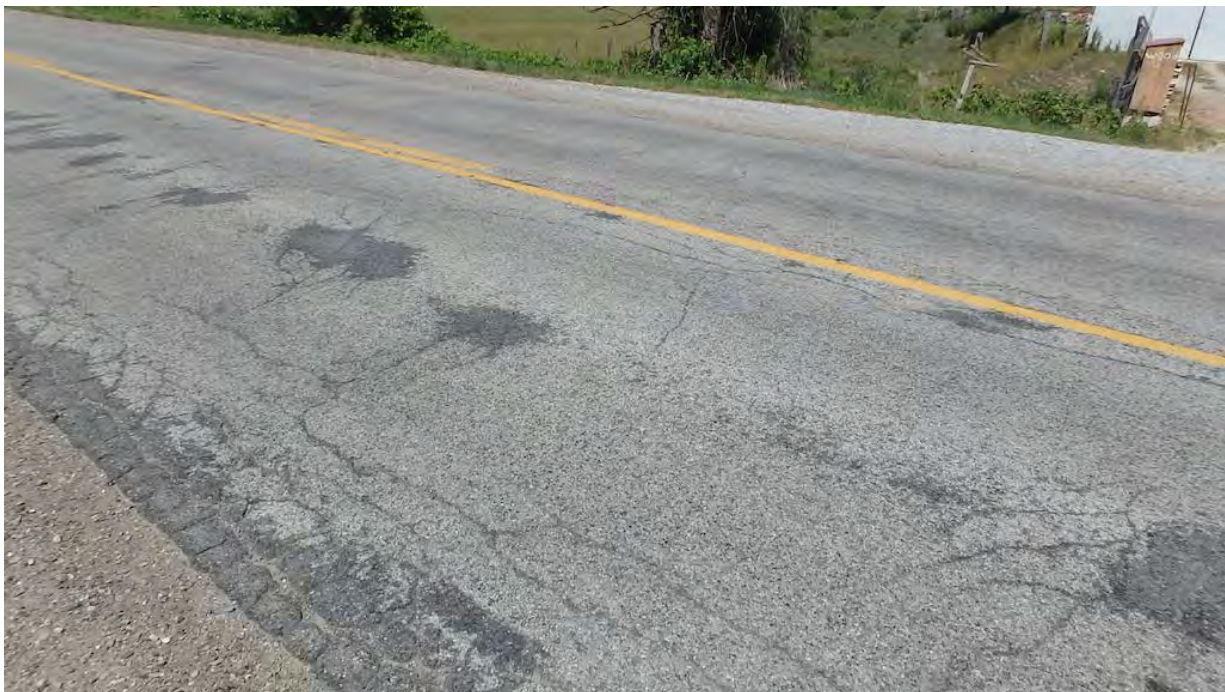
Figure 10 Rutting and Map Cracking on Wearing Surface
