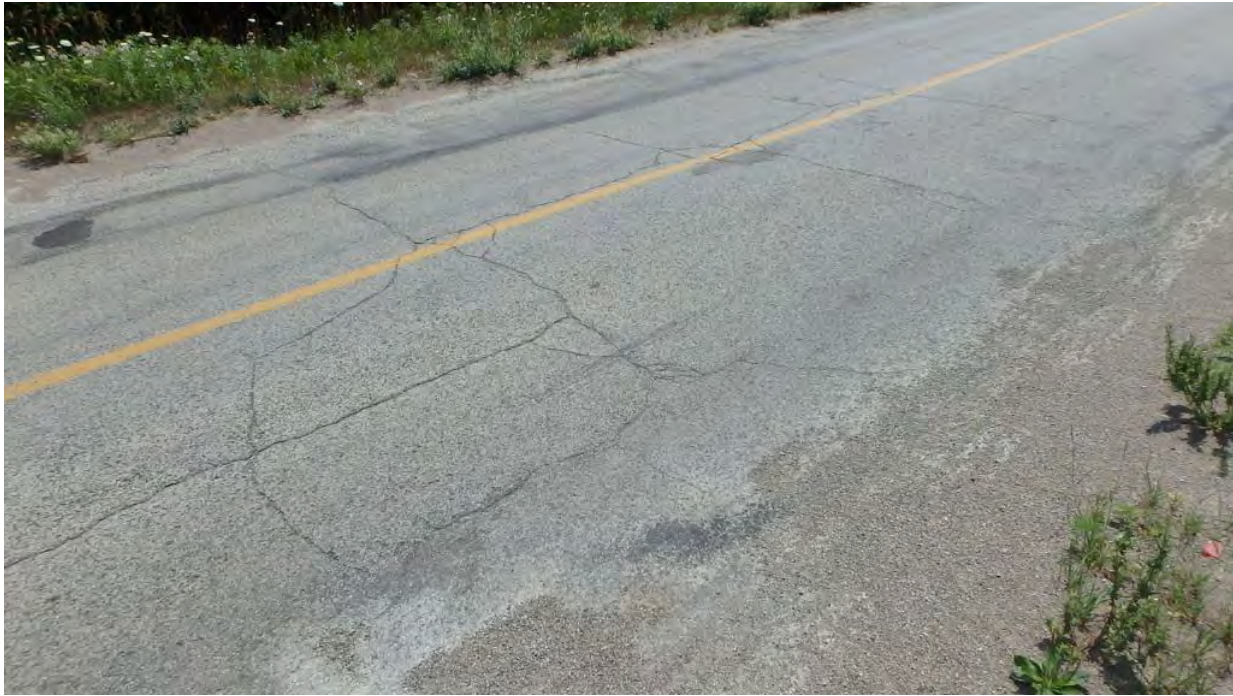
Figure 13 Cracking & Settlement at Road Edges at Culvert
