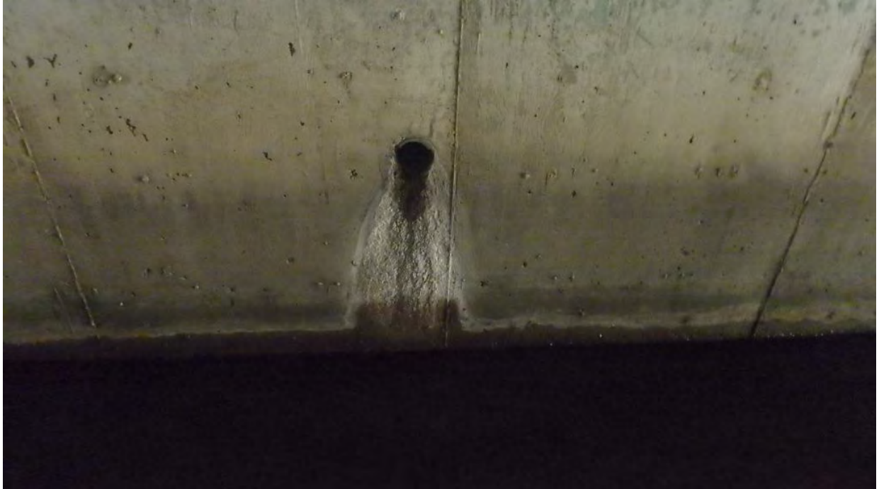
Figure 12 Deterioration at Weeping Holes
