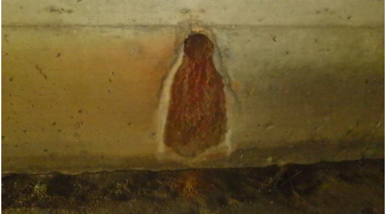
Figure 10 Weeping Holes Full of Debris
