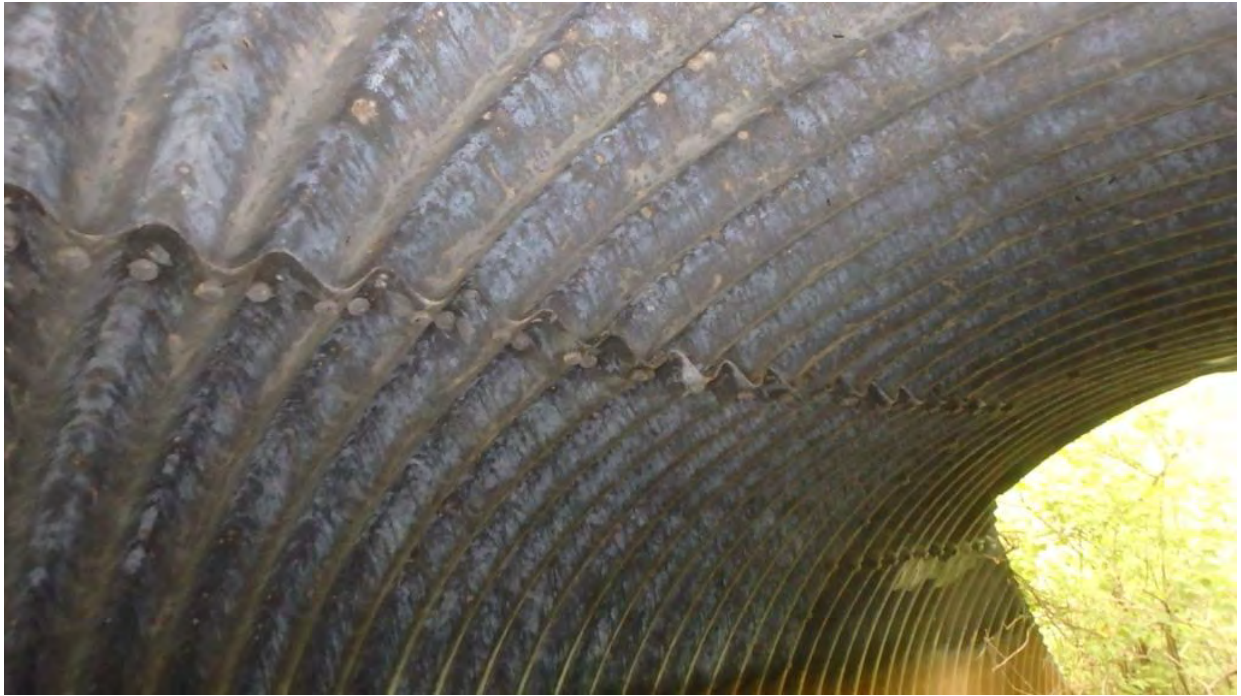
Figure 9 Deflection at Joint
