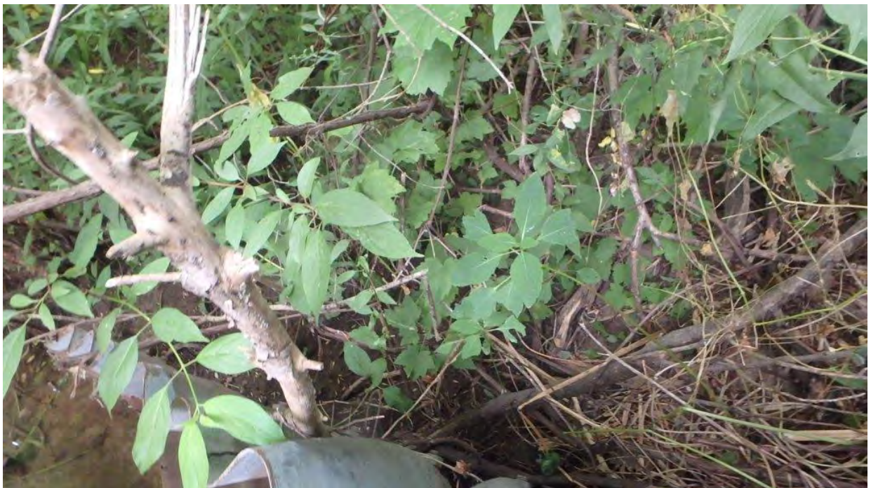
Figure 12 Erosion at North Quadrants
