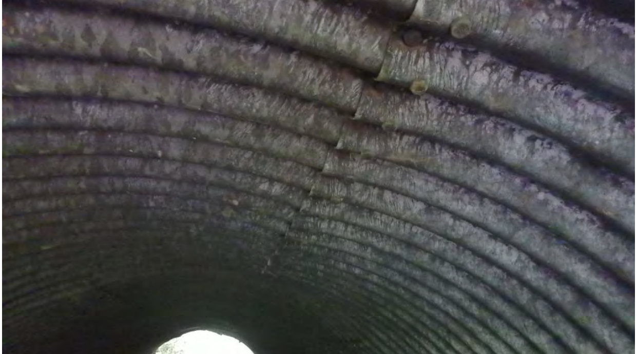
Figure 10 Deflection in Multiplate Joint
