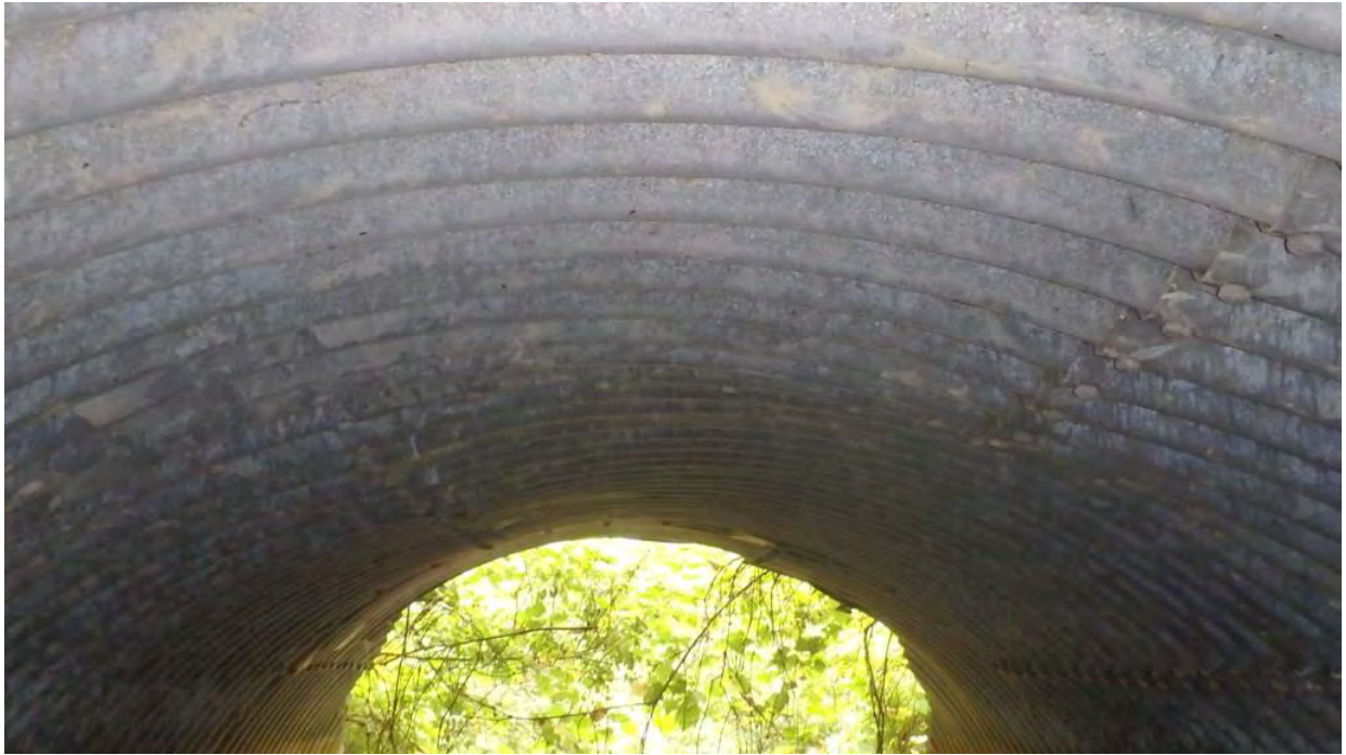
Figure 11 Deflections in Multiplate Joints at North End
