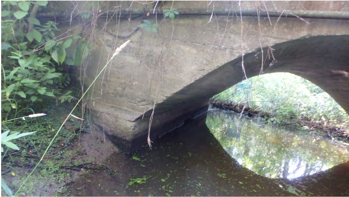
Figure 7 Deterioration of Walls
