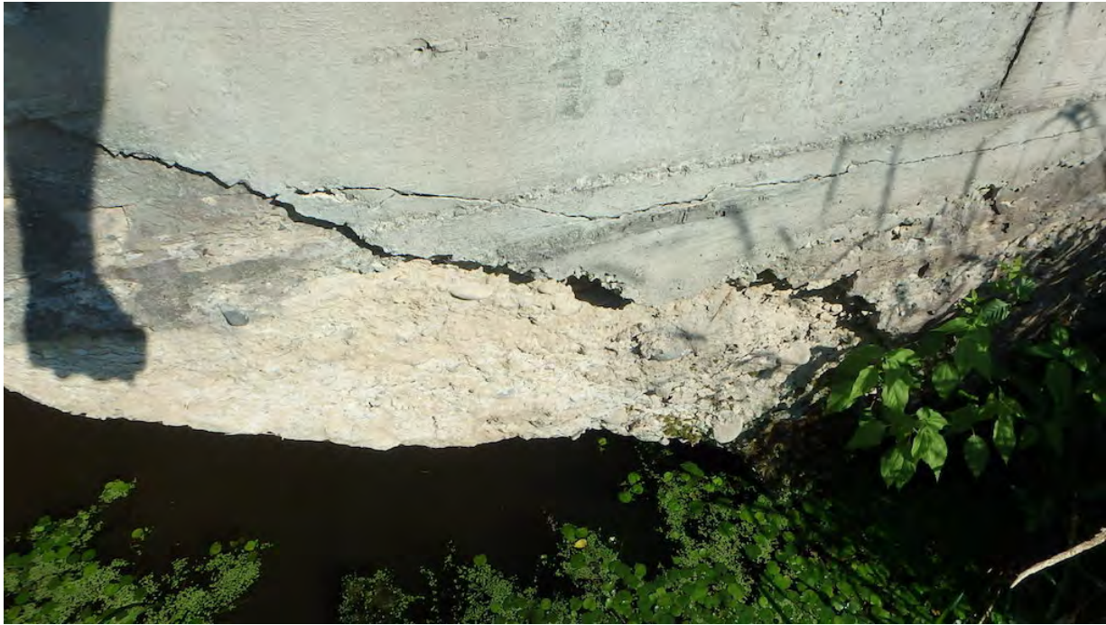
Figure 7 Deterioration of Fascia
