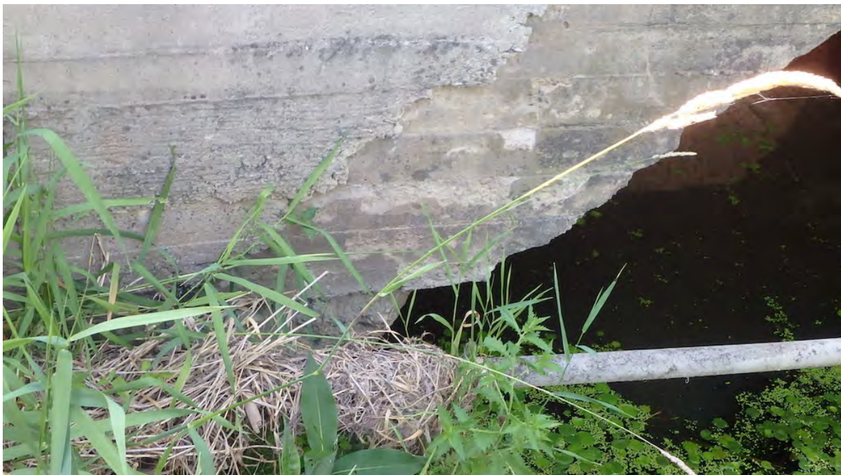
Figure 8 Deterioration of Wingwall
