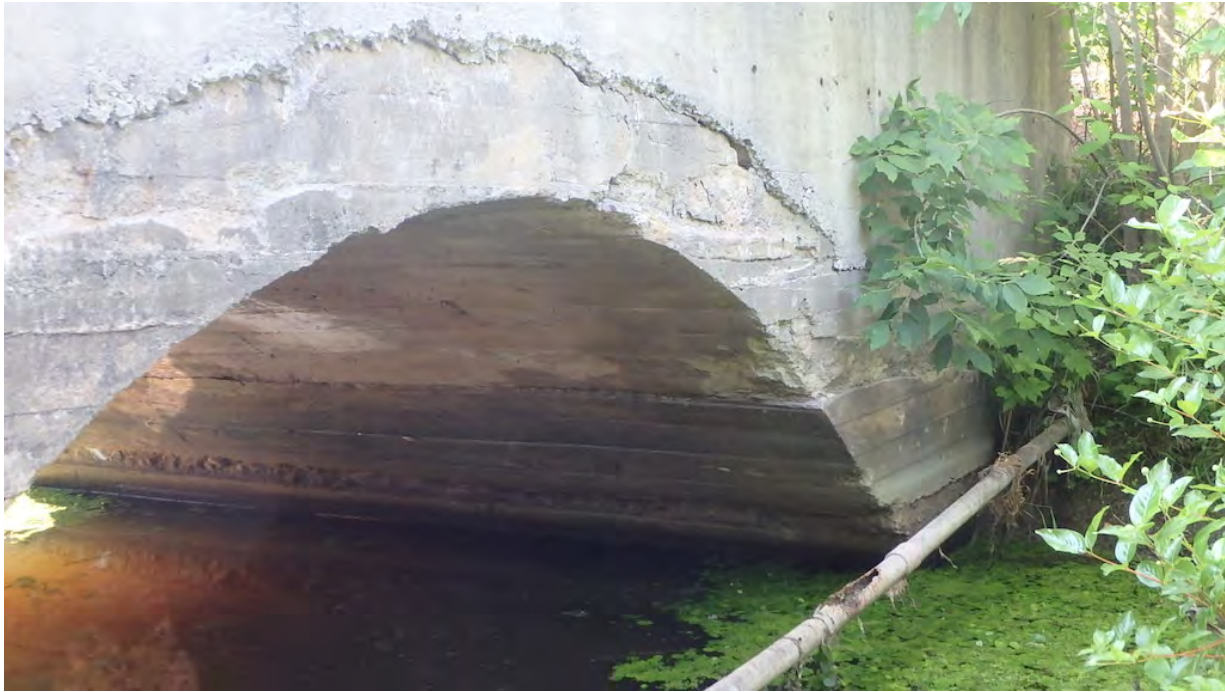
Figure 9 Transverse Crack Along Soffit
