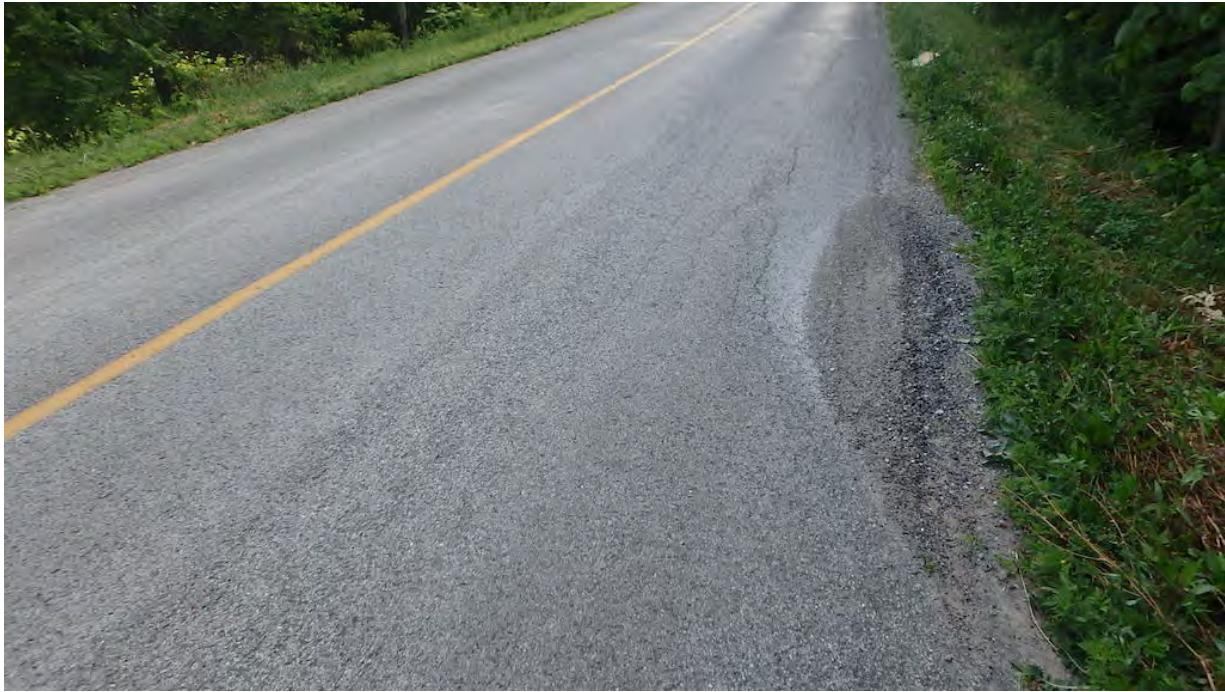
Figure 7 Minor Settlement and Cracking at Road Edges
