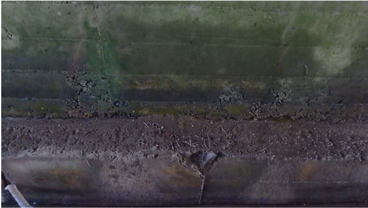
Figure 9 Honeycombing on Footing and Walls
