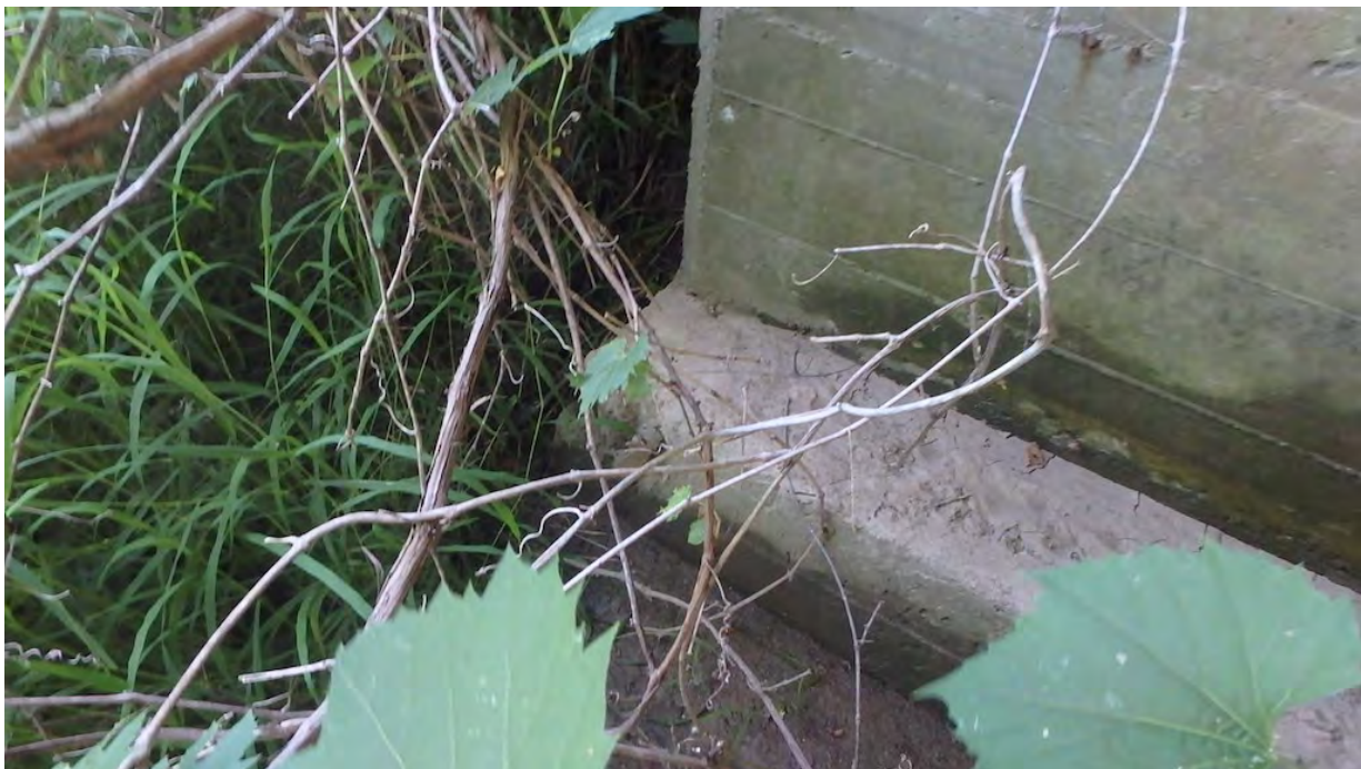
Figure 10 Spall on Footing at Southwest Corner
