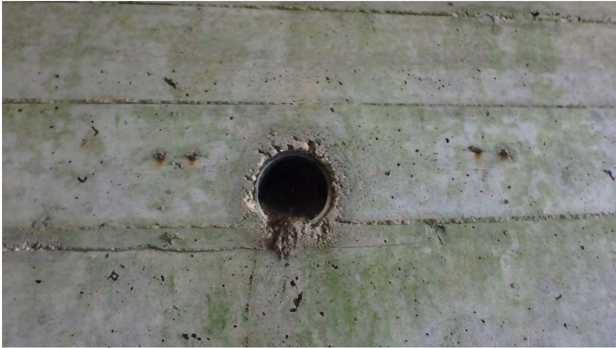
Figure 11 Weeping Holes Plugged with Debris
