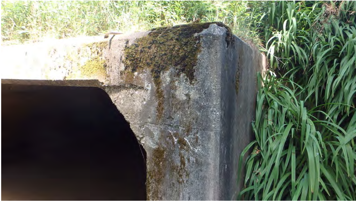
Figure 9 Minor Scale and Construction Joint Deterioration
