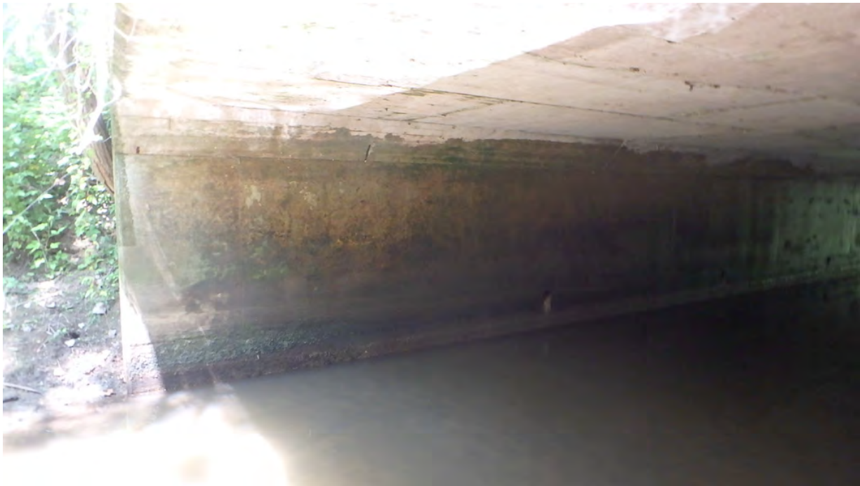
Figure 8 Staining and Wetness on Wall
