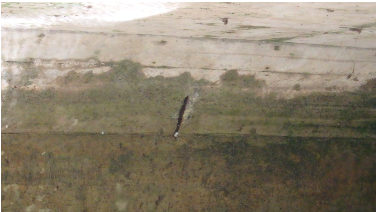
Figure 10 Popout with Exposed Rebar
