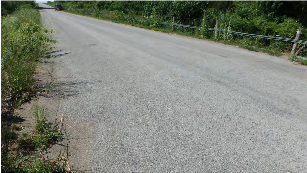
Figure 9 Minor Settlement at Structure Edges
