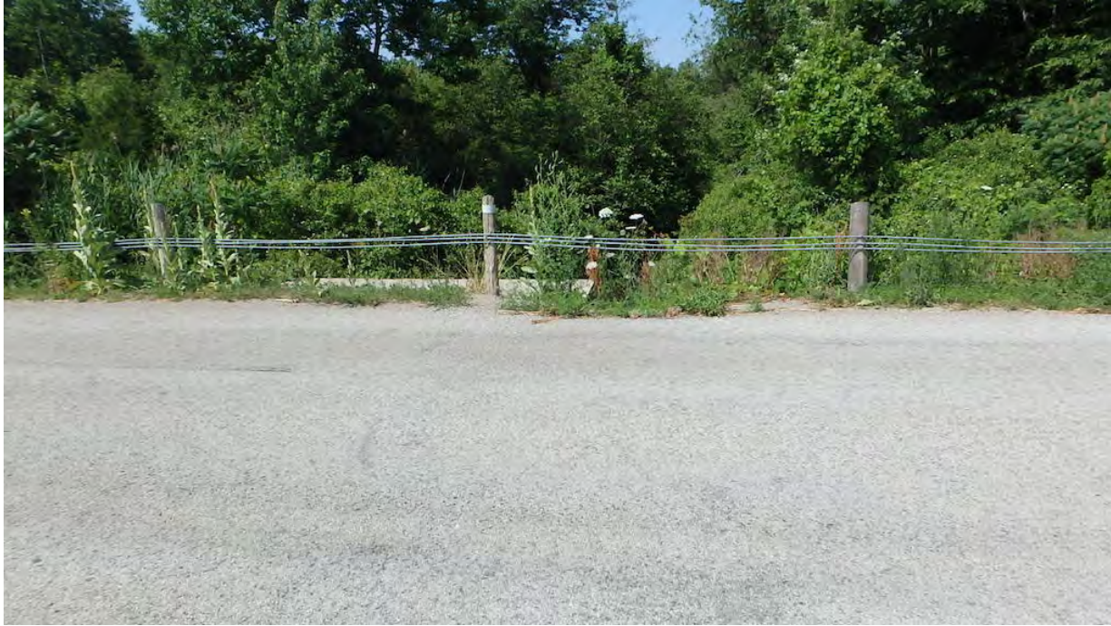
Figure 11 Loose Guiderail Cables
