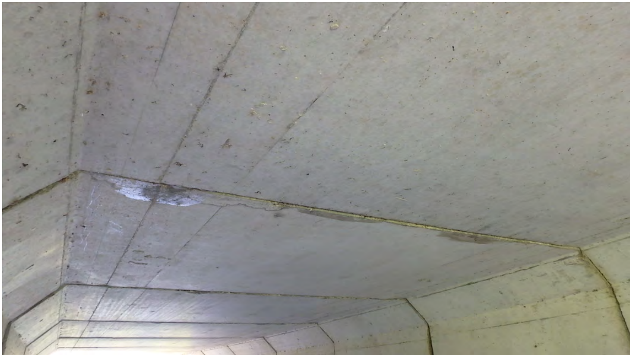
Figure 8 Staining on Soffit
