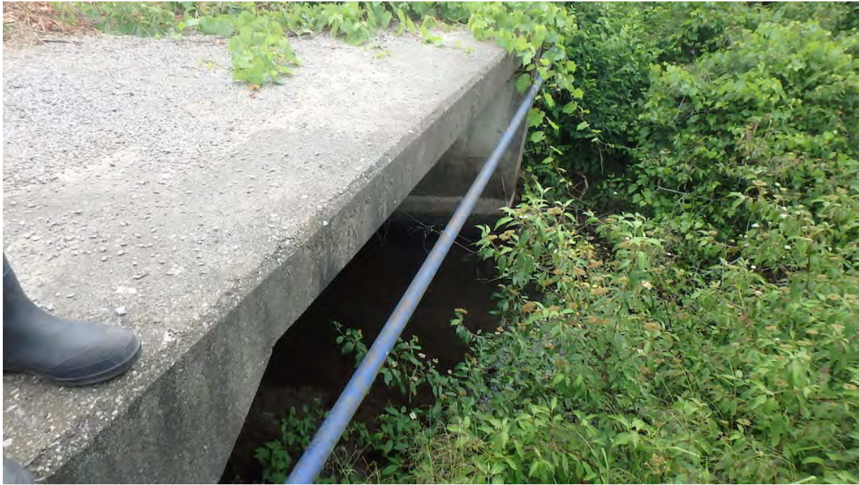
Figure 9 Gas Line on Fascia
