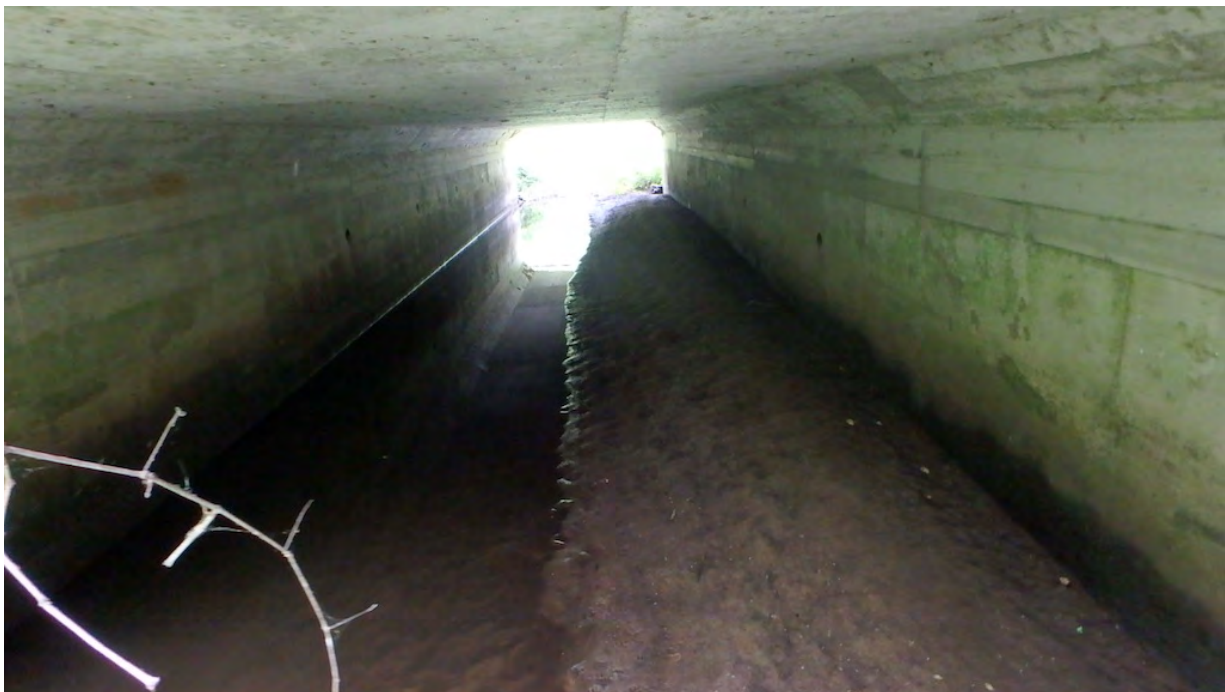
Figure 8 Barrel, Note Buildup of Material Along East Wall
