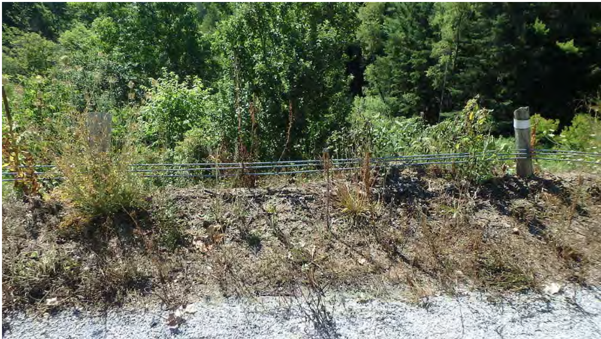
Figure 6 Three Cable Guiderail at South, Loose Cables
