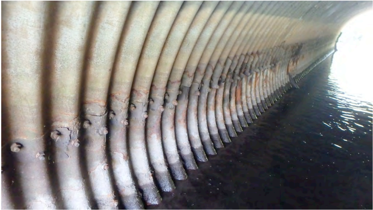
Figure 9 Corrosion at South Wall
