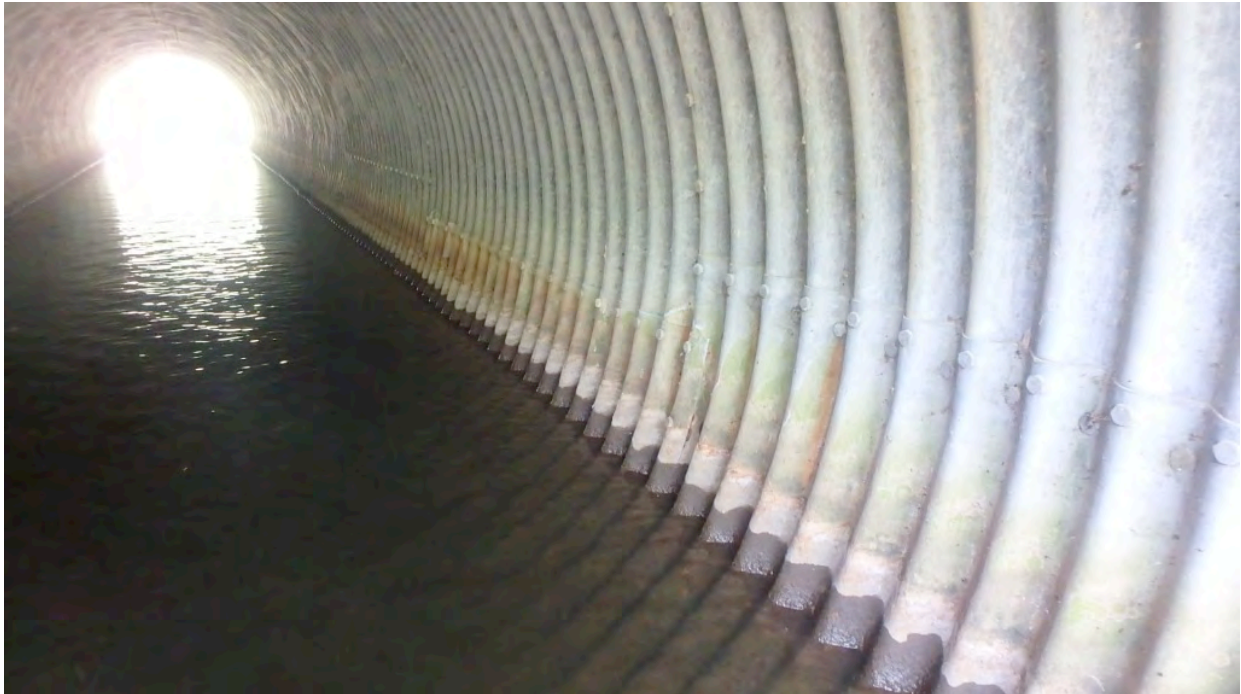
Figure 8 Corrosion and Staining at Water Line
