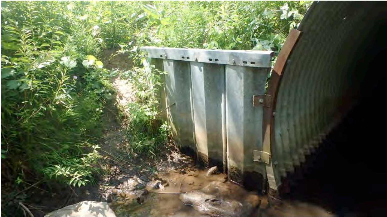
Figure 9 Retaining Walls at All Quadrants, Note Minor Erosion
