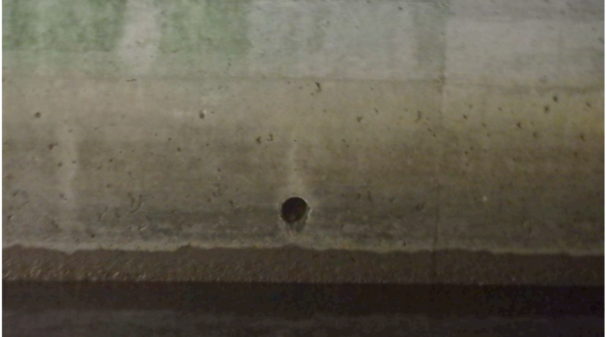
Figure 10 Narrow Crack at Weeping Hole
