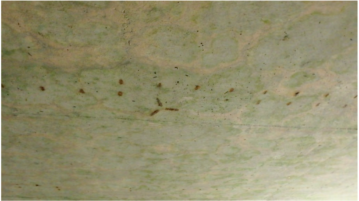
Figure 9 Exposed Reinforcing Ties
