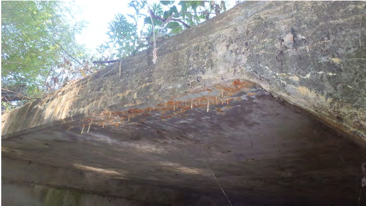
Figure 7 Delamination on South Fascia and Soffit
