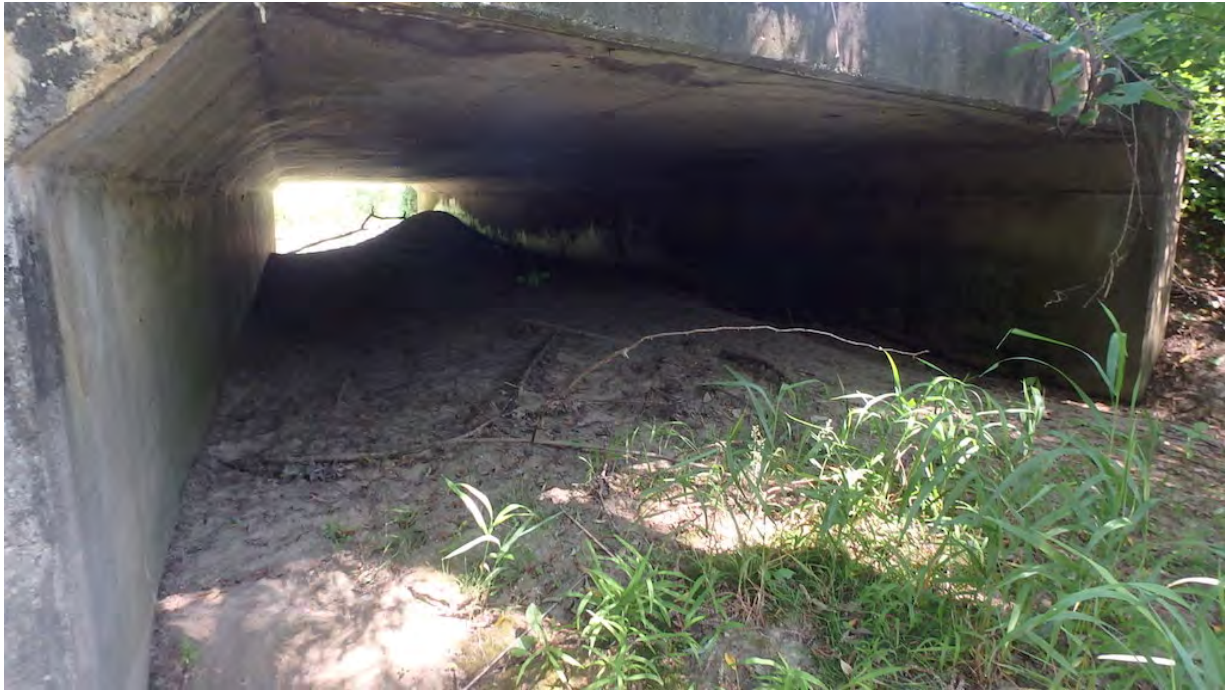
Figure 5 East Barrel, Note Fully Blocked with Sediment
