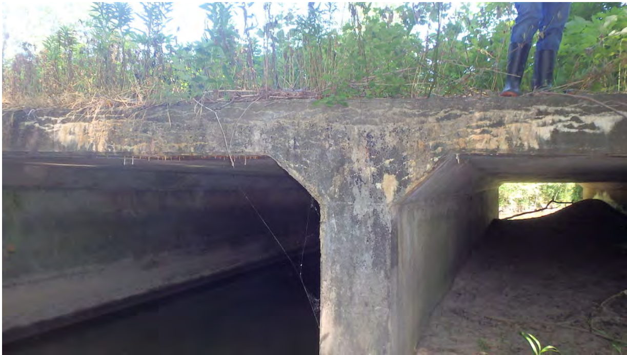
Figure 9 Map Cracking with Efflorescence on South Fascia
