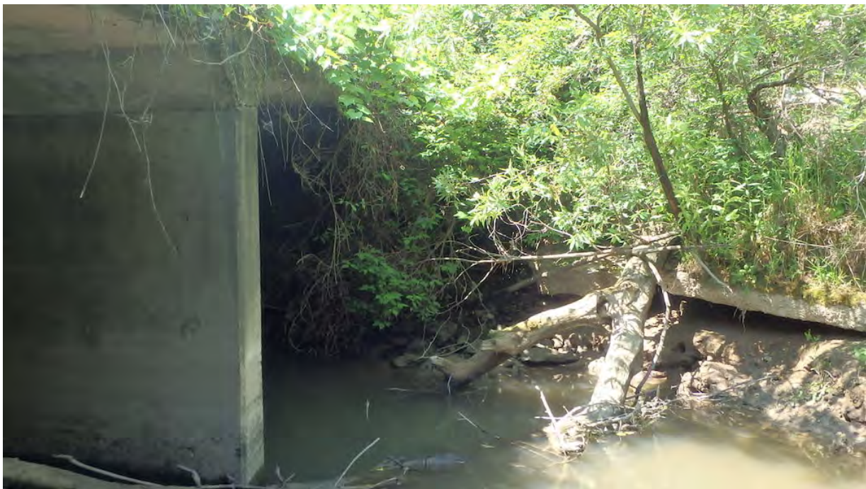
Figure 10 Overgrown at Quadrants
