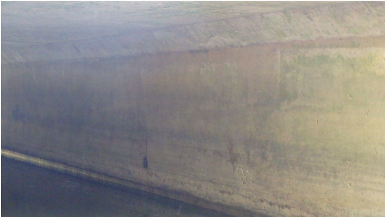
Figure 11 Vertical Crack in Centre Wall, West Barrel
