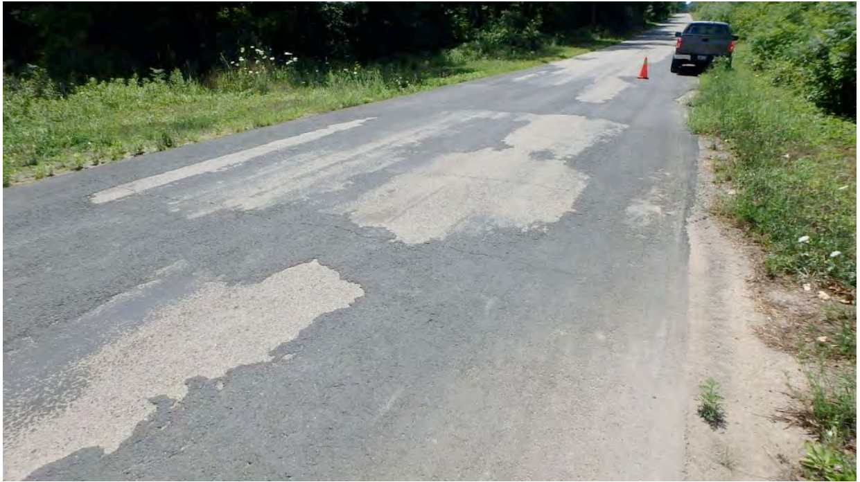
Figure 11 Settlement at Structure Edges Patched
