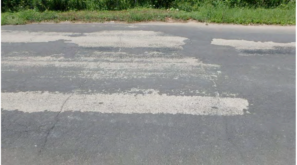
Figure 12 Transverse Cracks at Structure Edges
