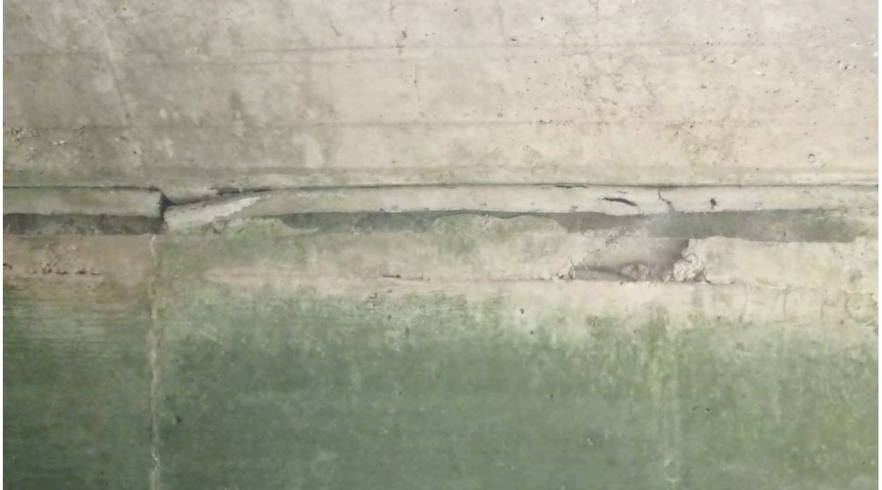
Figure 10 Minor Deterioration of Construction Joint
