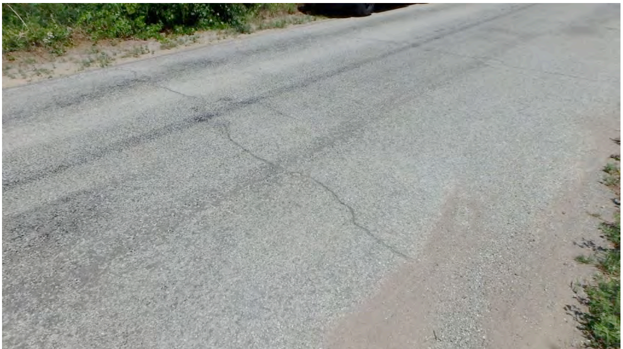
Figure 8 Transverse Crack in Wearing Surface
