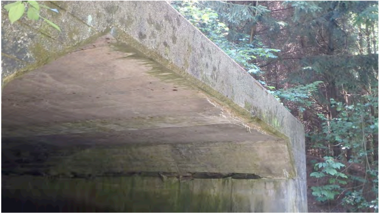
Figure 7 Efflorescence & Deterioration at Inlet Fascia
