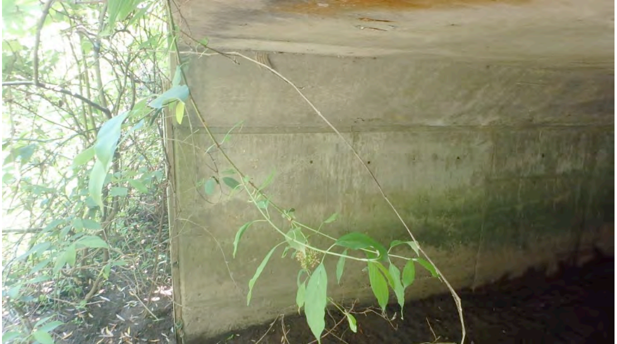
Figure 10 Minor Staining East Wall
