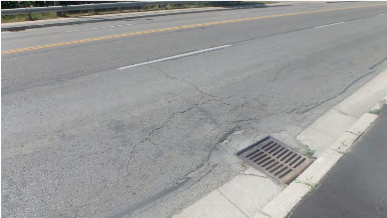
Figure 9 Longitudinal & Transverse Cracking throughout Wearing Surface
