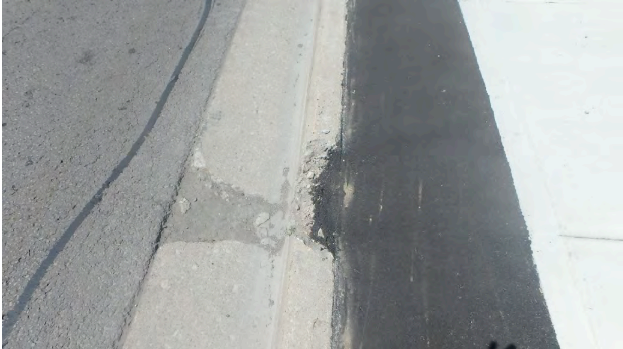
Figure 10 Spall in East Curb
