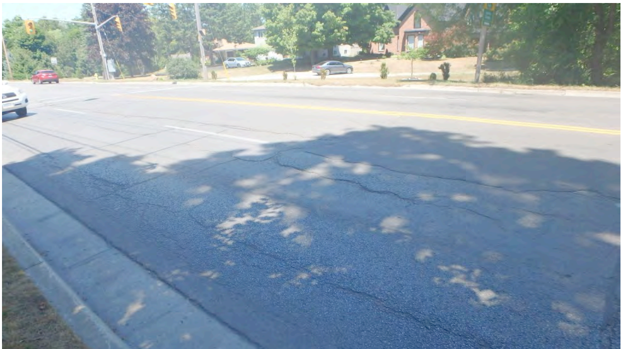
Figure 12 Longitudinal & Transverse Cracking throughout Wearing Surface
