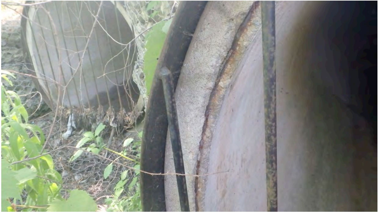
Figure 11 Small Spalling with Exposed Rebar on Pipe Exterior
