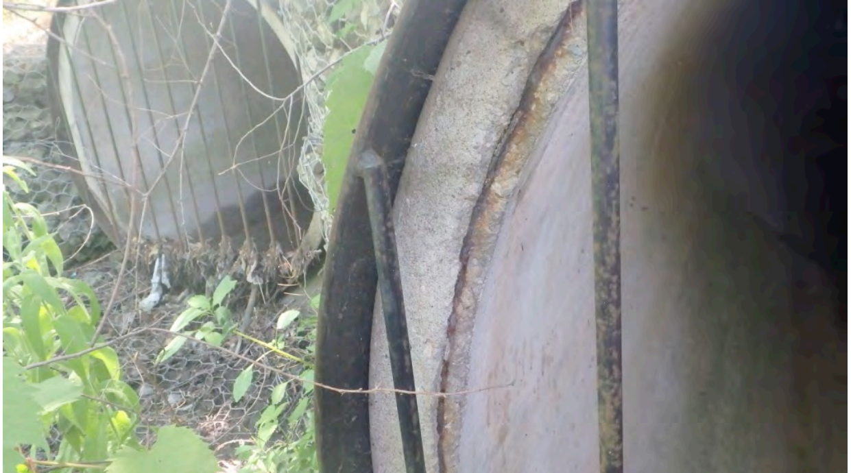
Figure 8 Small Spalling with Exposed Rebar on Pipe Exterior
