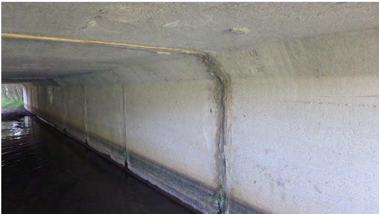
Figure 8 Typical Cracking and Deterioration of Parging at Joint
