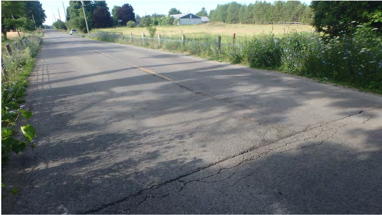
Figure 9 Transverse and Longitudinal Cracking in Wearing Surface
