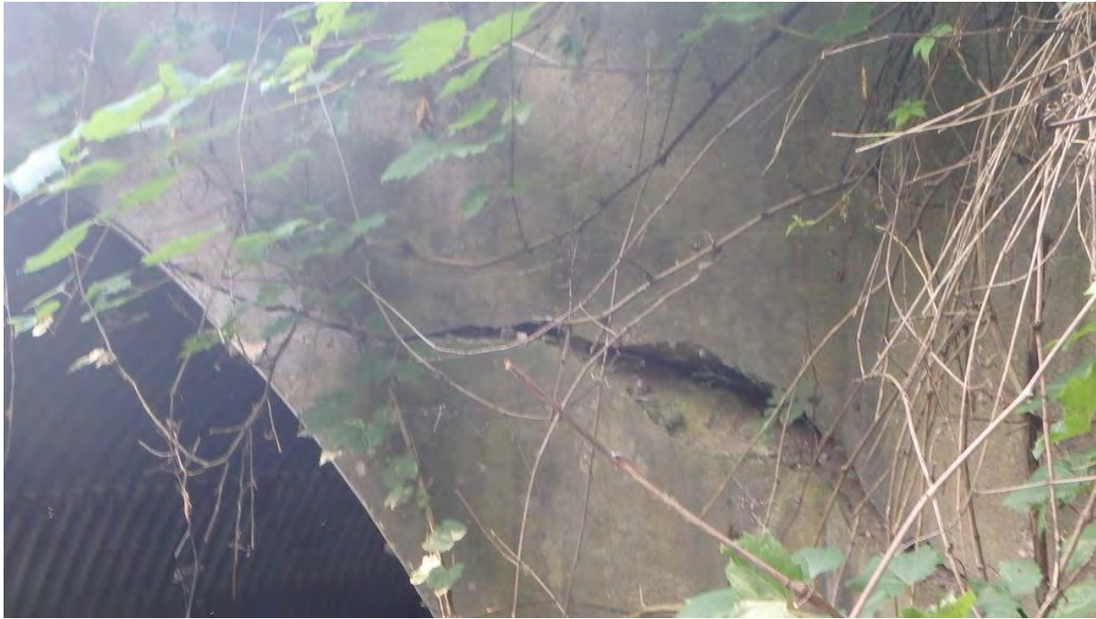
Figure 9 Large Crack in North Fascia
