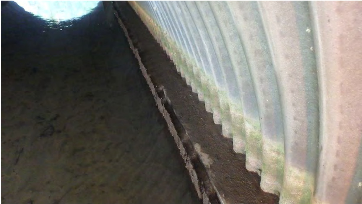
Figure 11 Typical Corrosion at Waterline in Barrel
