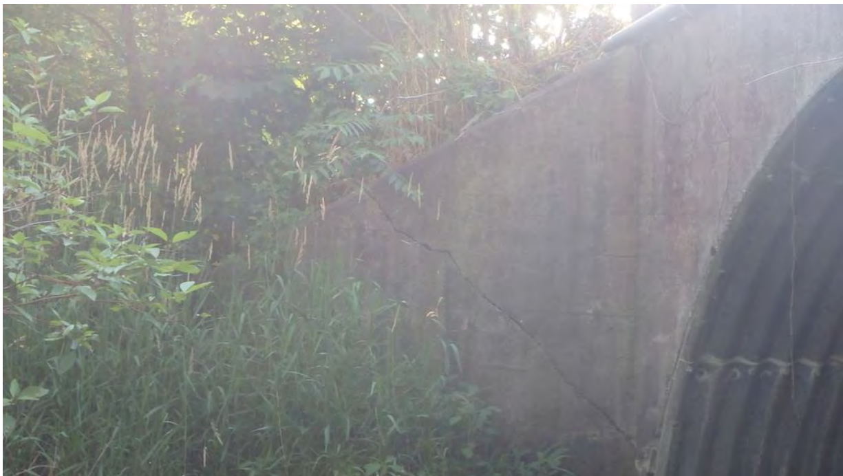
Figure 10 Large Crack in Northeast Wingwall
