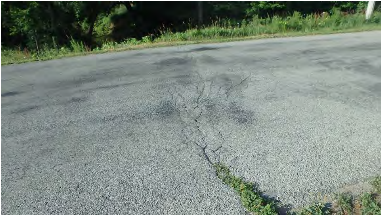
Figure 12 Transverse Cracking in Wearing Surface
