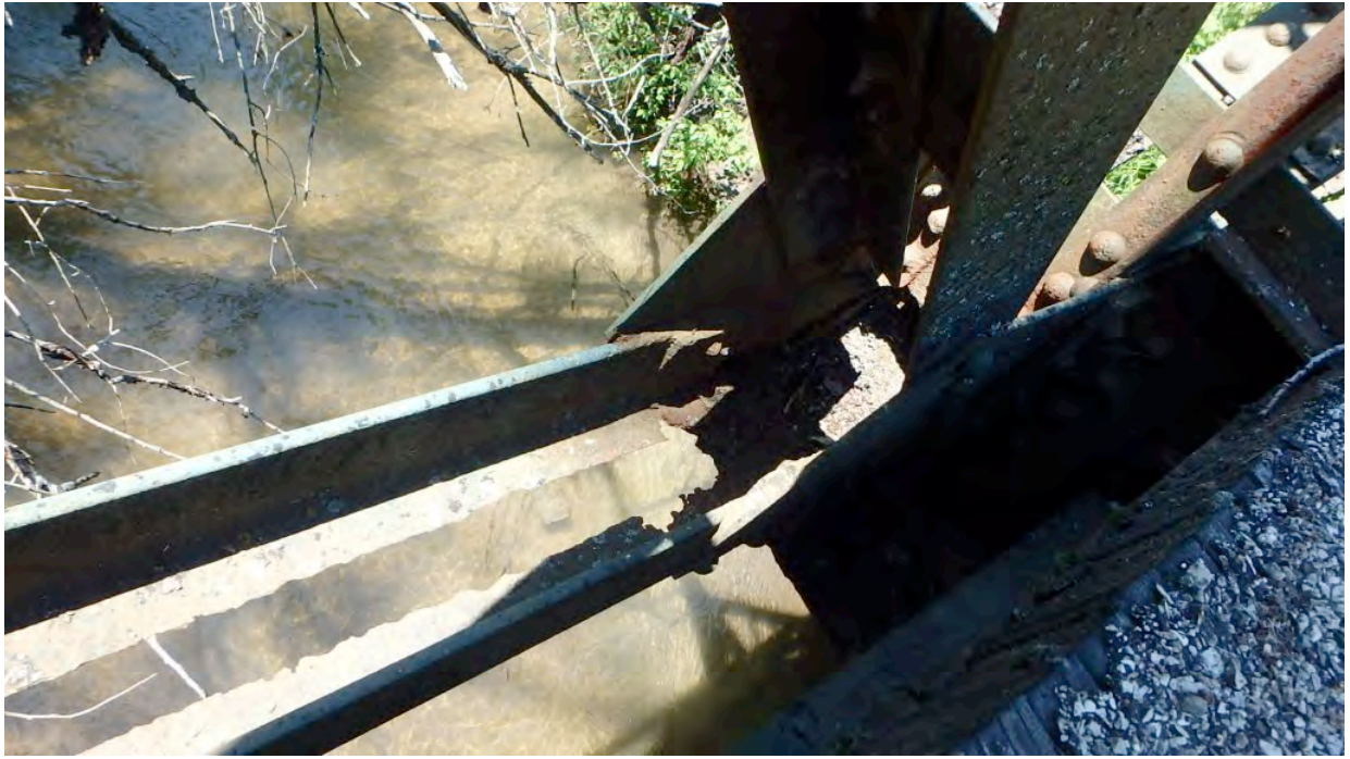
Figure 7 Severe Corrosion of Bottom Chord
