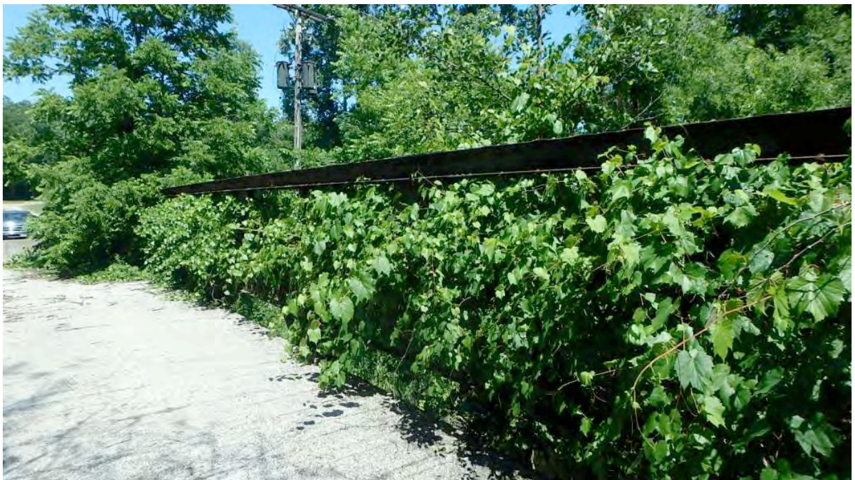
Figure 6 South Truss Overgrown
