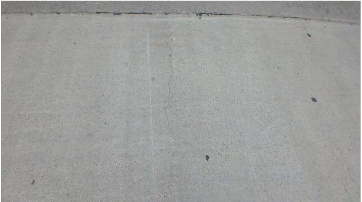
Figure 13 Longitudinal Crack in Concrete Deck Wearing Surface
