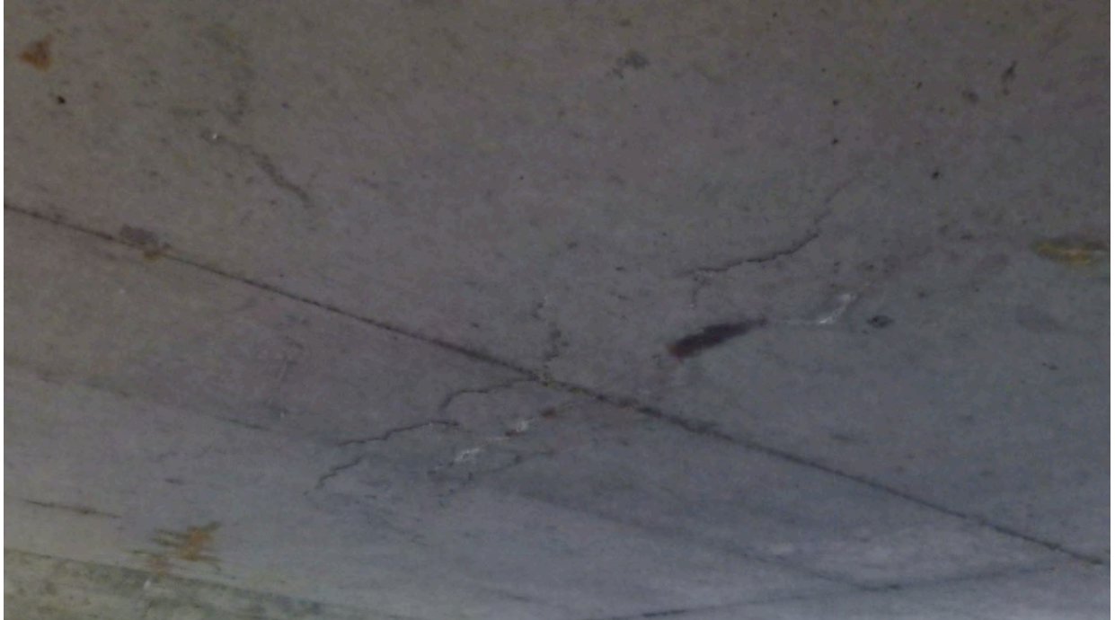
Figure 8 Crack on Culvert Soffit
