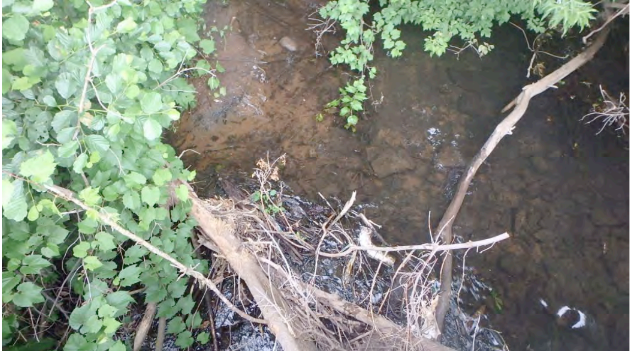
Figure 14 Debris at Outlet
