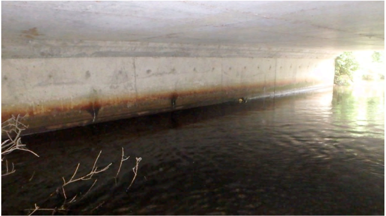
Figure 9 Staining on Culvert Walls at Waterline
