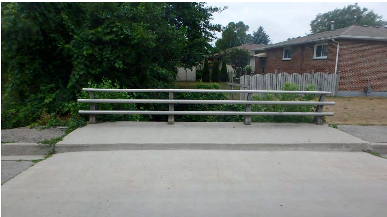
Figure 12 Slight Bend in Top Rail of North Barrier
