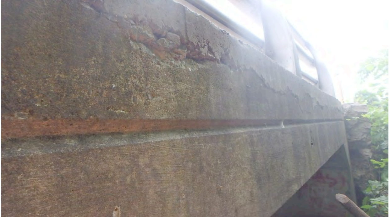
Figure 10 Spall at Construction Joint
