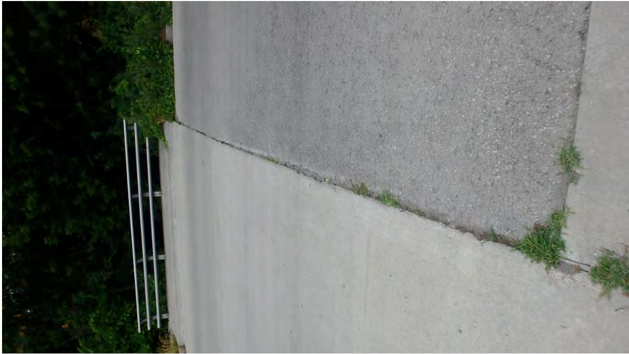
Figure 11 Asphalt Approach Slightly Lower than Concrete Deck
